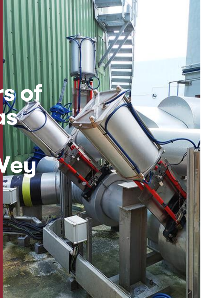
Wey MFC DN 300 knife gate valves in the outside area of the system.
