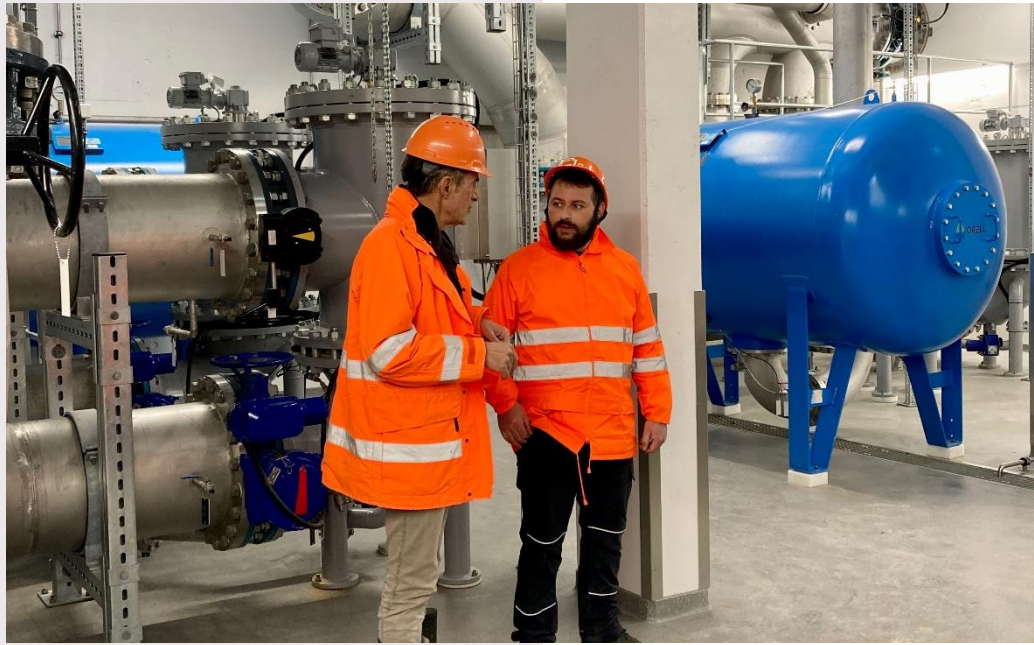
Inside the new pumping station on the shores of Lake Geneva
